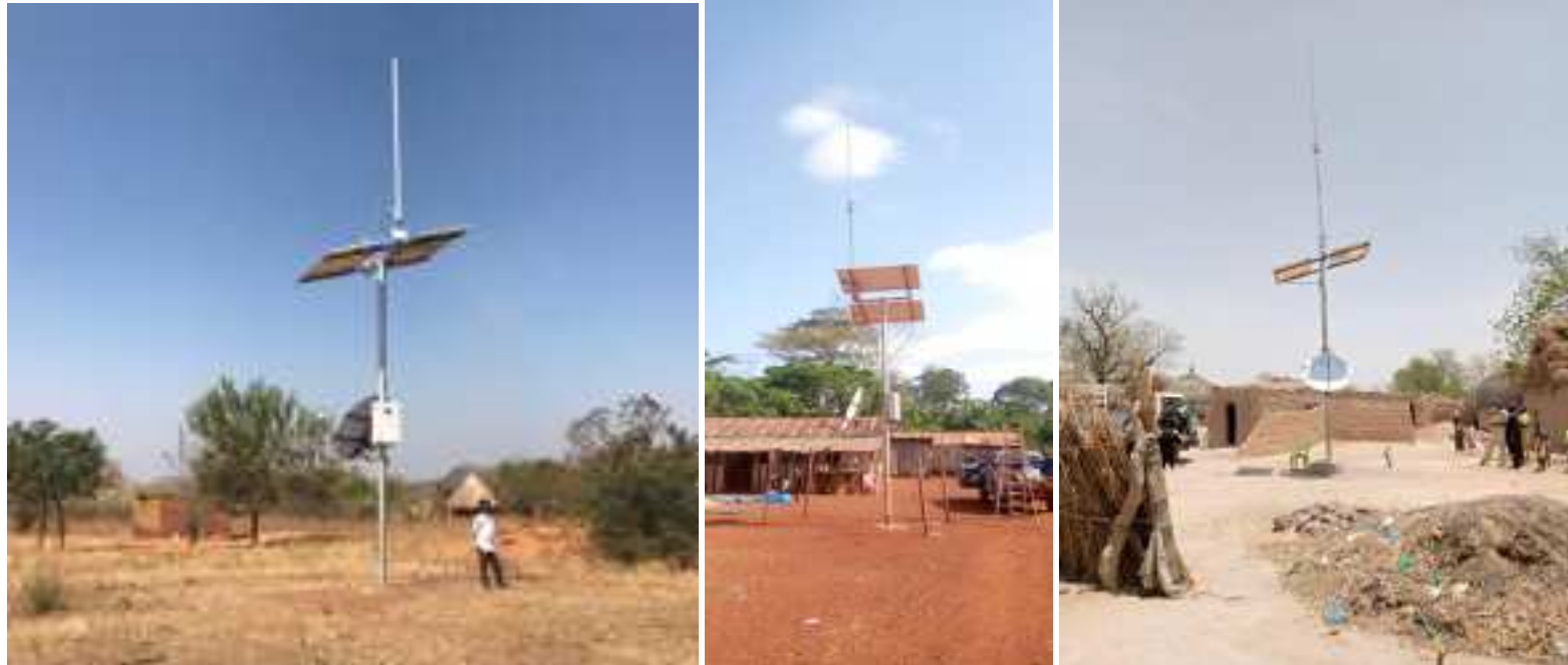
Box 4 figure: Remote Africa Mobile Networks AMN small site deployments
