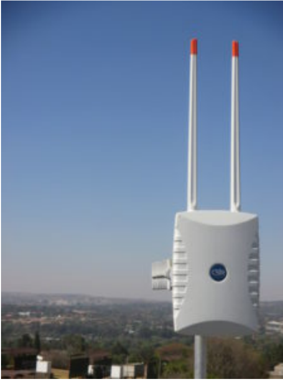
Fig. 1: A CSIR High-Performance WiFi node with a UHF Whitespace antenna provides local coverage and long-distance backbone capability.
